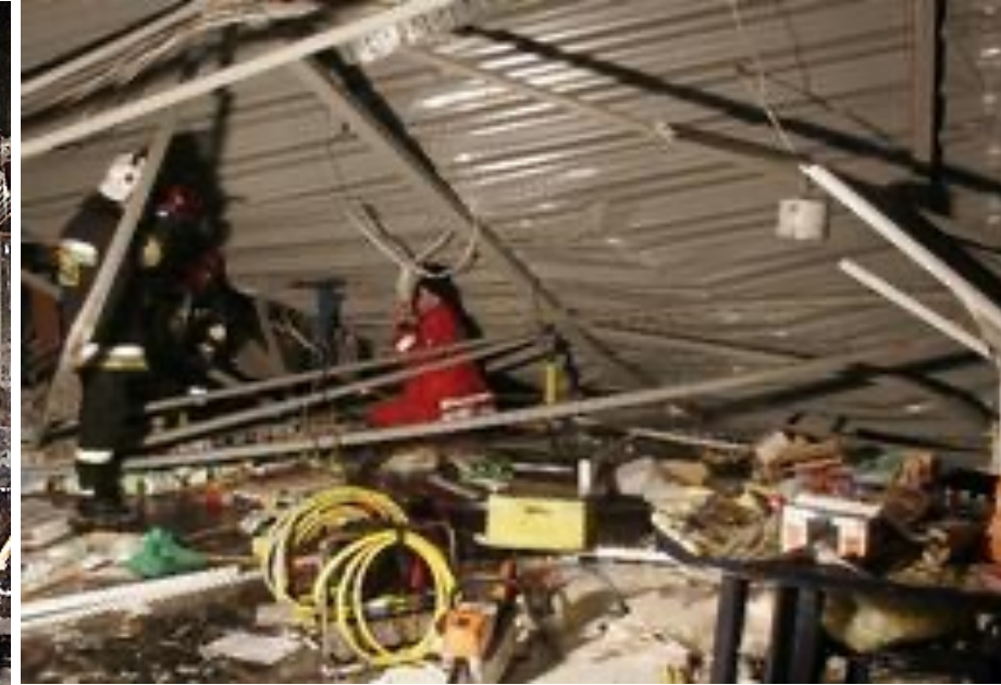
Exhibition Hall, Katowice in Poland, Jan.28th,2006, 65 dead, 170 injured Completed in 1974
