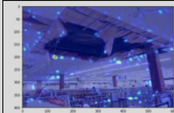
Saliency map to the ceiling image (damaged)
