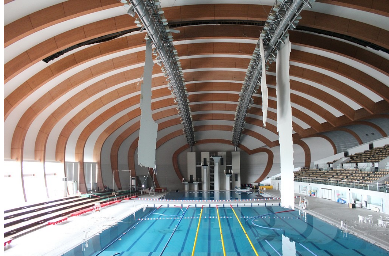
Ceiling fall in a swimming pool, July 2013
